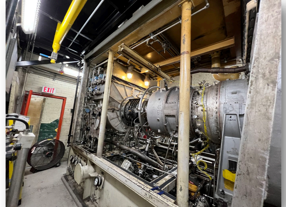
Natural Gas Cogen at CED that generates a consistent ~5.5 MVA (up to 6.4 MVA).
