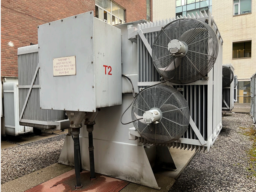
Largest transformer rating is a 4 MVA @ 13.8kV:4.16kV (we have 4 of these).
